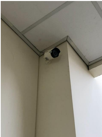
Surveillance camera (CCTV)
